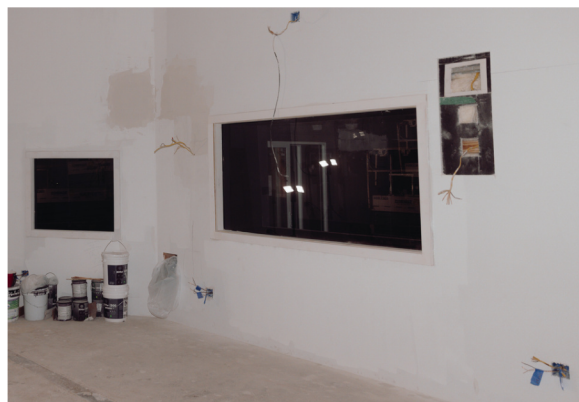
Photo: Main Sound Room looking at Control Room Window.
