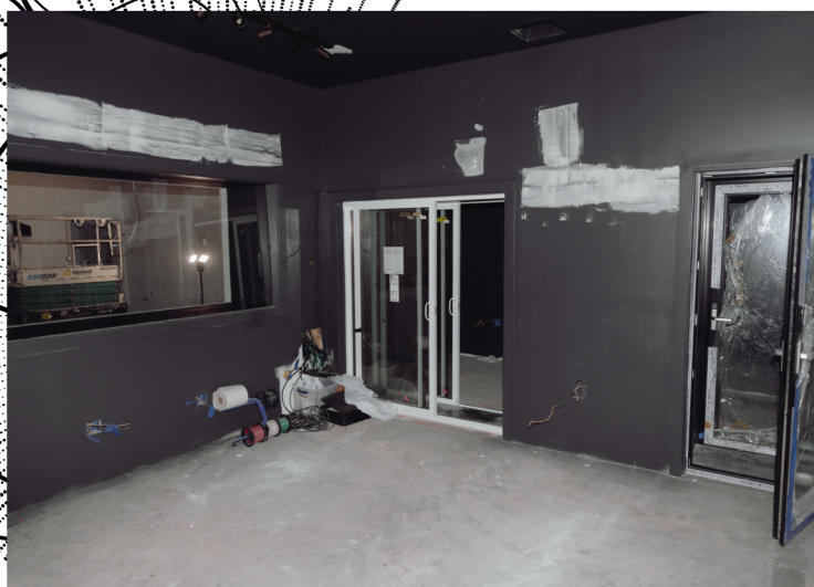
Photo: Sound-Proof Control Room w/ two smaller studio rooms adjacent
